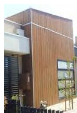
The board shows signs of lightening.
