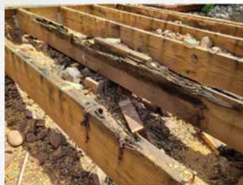
5 Year old deck frame
