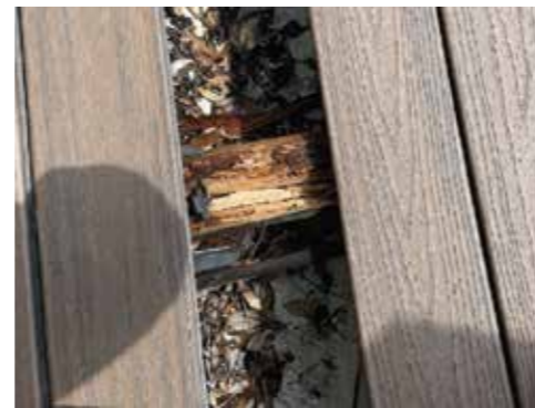
TIMBER FRAME FAILURE Trex Decking boards still in perfect condition but full frame replacement needed.
